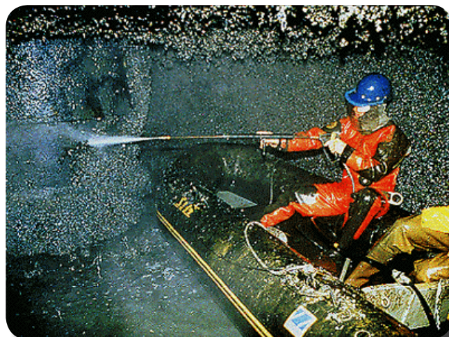
Pressure washing (aka “pigging”) is one method of removal of mussel colonies. Photo credit Zebra Mussel Information System, 2005.
