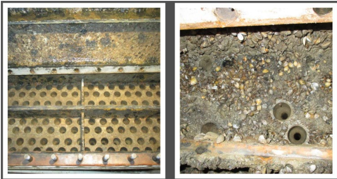
Figure 5. Clean generator air cooling tubes (left) versus generator air cooling tubes affected by Zebra Mussel biofouling.
