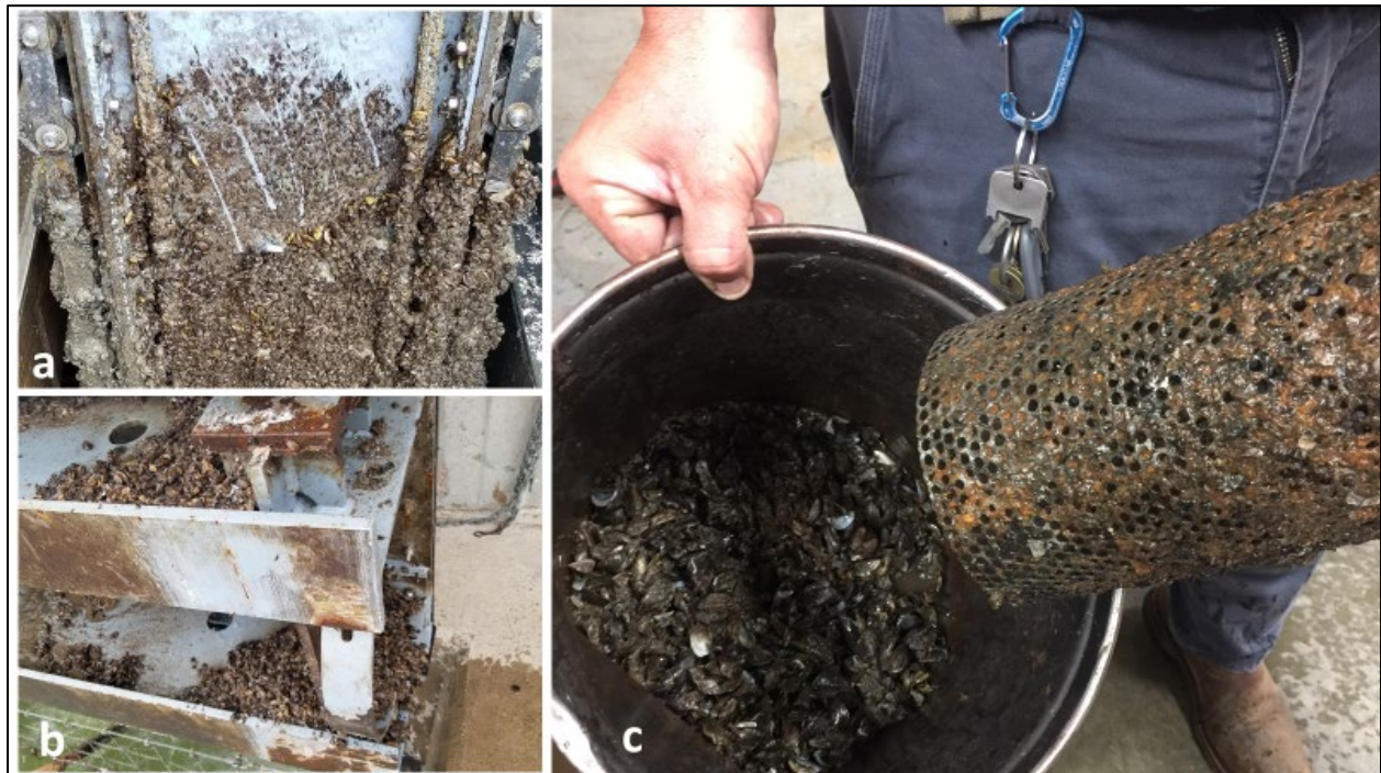
Figure 4. Zebra Mussel biofouling of water intake gate (a), spillway stop (b), and raw water booster pump strainer (c).
