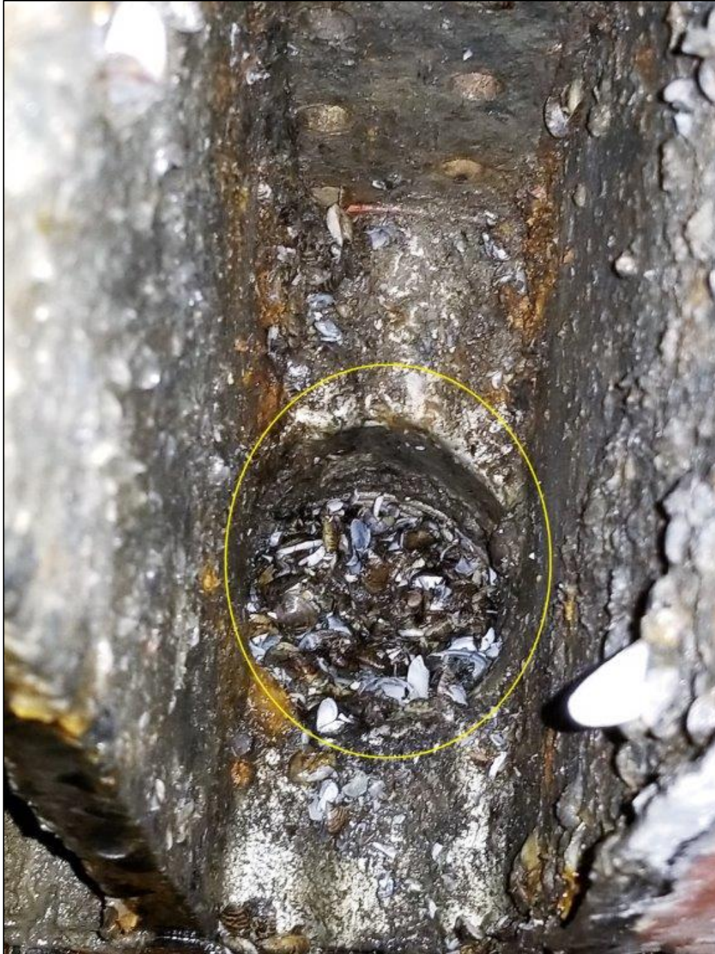
Figure 6. Air cooler tube plugged with ZM shells.
